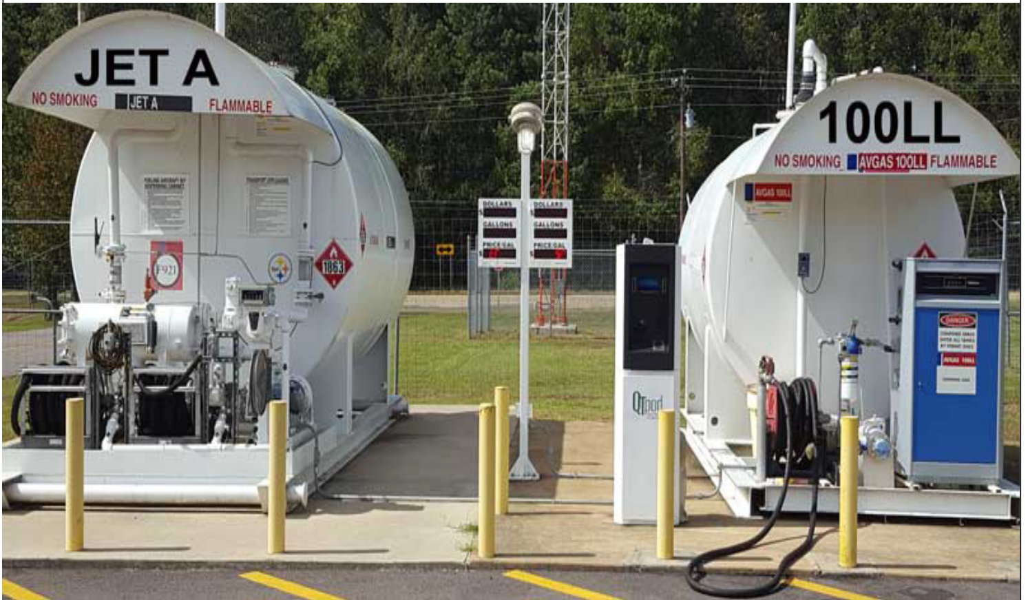
Fuel Station - Jet A and 100LL
